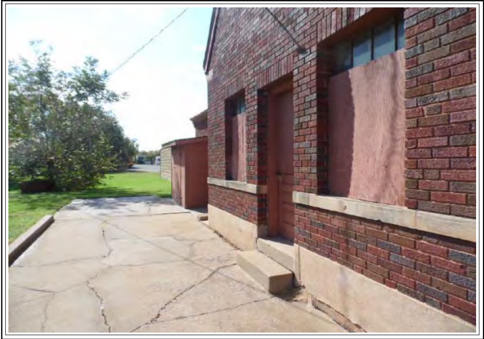
Boarded windows, unsure of condition
