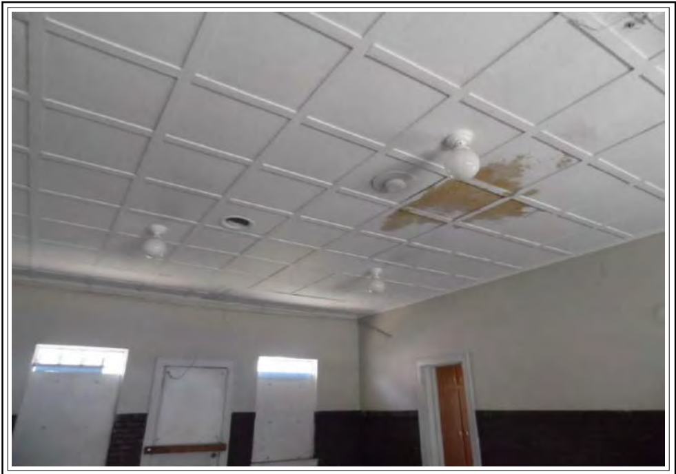
Ceiling needs painted
