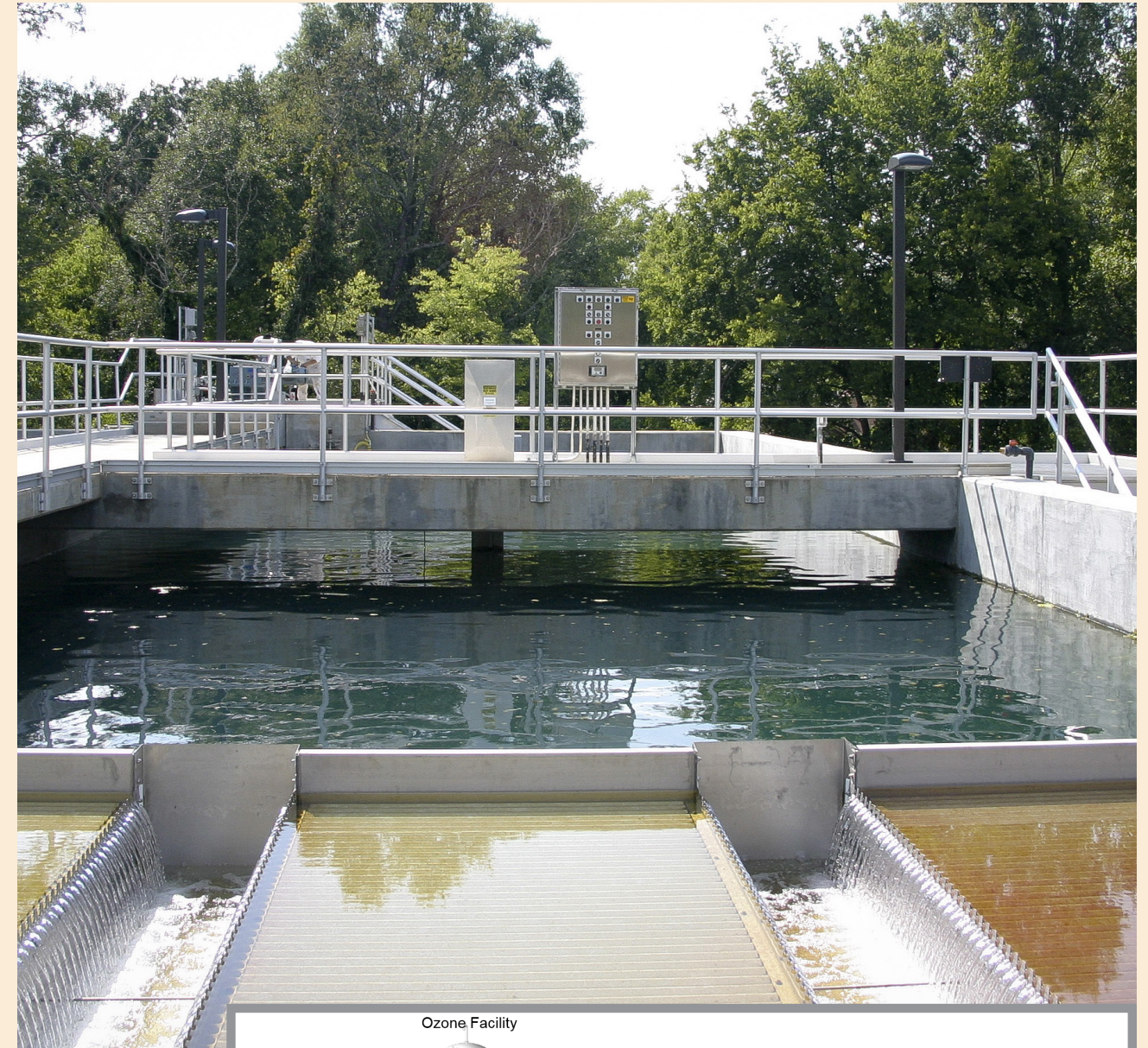
Above: Water treatment plant sedimentation basin
