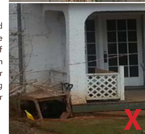
A well-maintained foundation not only adds to the overall character of your building, but ensures structural integrity.
