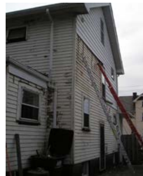
Rehab in process: Removal of aluminum to reveal historic wood siding still in good condition.
