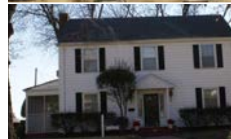
Many Colonial Revival style homes have side wings. These wings can usually be converted to rooms or porches without affecting building character.
