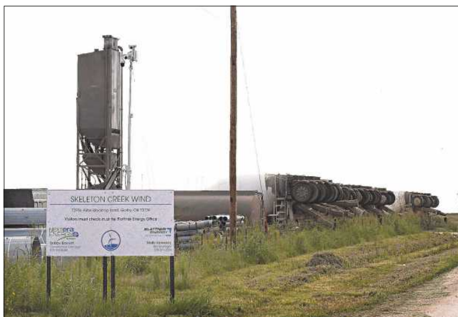
An on-site concrete batching plant for the Skelton Creek wind power project is located near Goltry. (Billy Helton / Enid News & Eagle)
