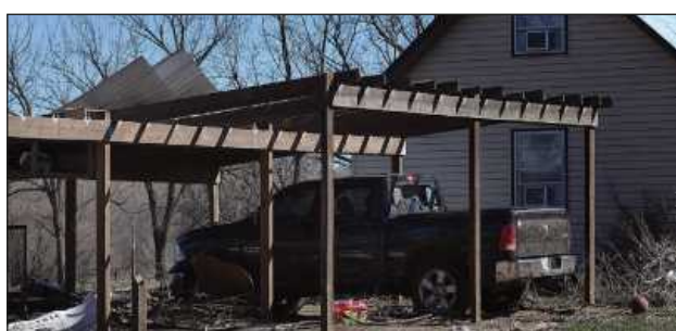
The back patio and balcony at 2000 Norman Road in Enid was damaged during Sunday's storm. (Billy Hefton / Enid News & Eagle)
