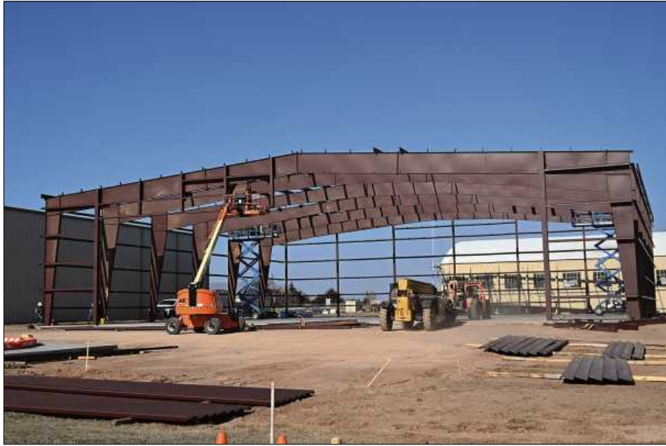
Construction continues on a new hangar at Enid Woodring Regional Airport. (Billy Hefton / Enid News & Eagle)
